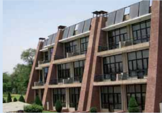
Jain Solar Water Heaters installed at TERI in New Delhi
