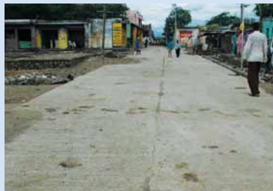
Concrete roads and drainage are amongst a few of the many social initiatives taken at Wakod by Jains
